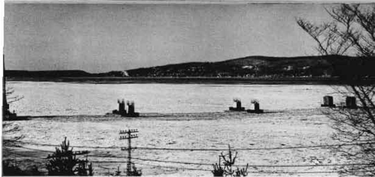
Ice that piled up against the piers was a major difficulty in construction of the bridge
